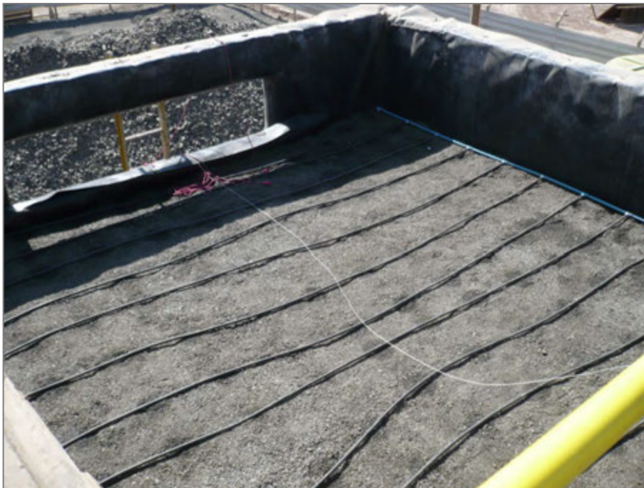
Irrigation Pipe 400 mm間隔
